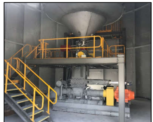
Lime Systems designed and supplied bin activator and access structure.
