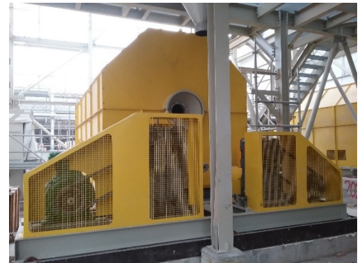
2.3m Diameter Lime Slaking Mills, fully enclosed for safety
