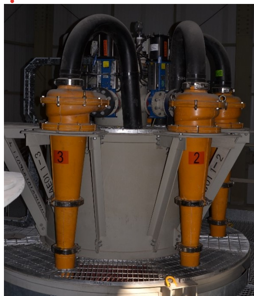
Hydrocyclone clusters for lime slurry particle size classification
